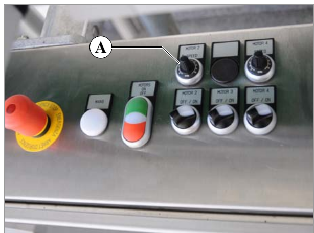
[17] Potentiometer (A) on the switch cabinet of the motor controller (example: NOVEXX Solutions, AMC Series).
