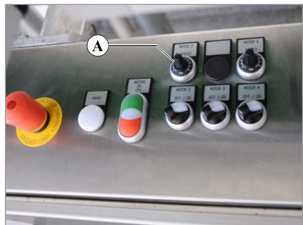
[14] Potentiometer (A) on the switch cabinet of the motor controller (example: NOVEXX Solutions, AMC Series).
